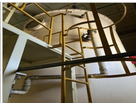
[Scrubbers in the Eonhaa Plant]
